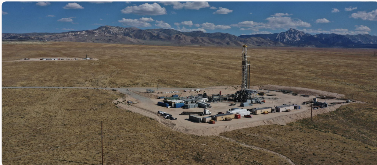
The Cape Station plant in Beaver County, Utah, will have a capacity of 400MW over its first two phases
